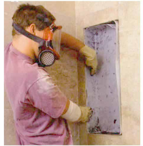
Fabric is pressed into the wet liquid. After the inside of the shampoo niche is coated with a latex-rubber liquid, a nonwoven polyester fabric is pressed into the liquid.
