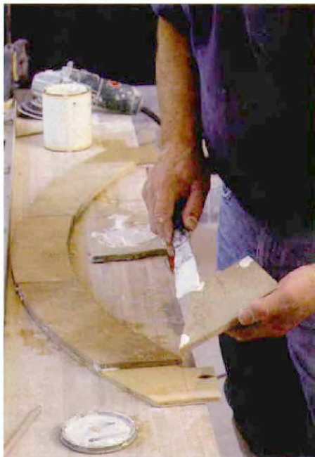
Cut tiles are glued temporarily to the template. After the tiles are cut, the author glues them to the template. Having the tiles aligned the way they will be installed makes it easier to keep the edge shape consistent.
