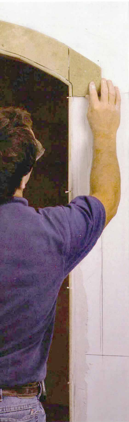
The arch goes up. Once the tiles are shaped and smoothed, they are installed on the wall, leaving the proper spacing for an attractive grout joint.
