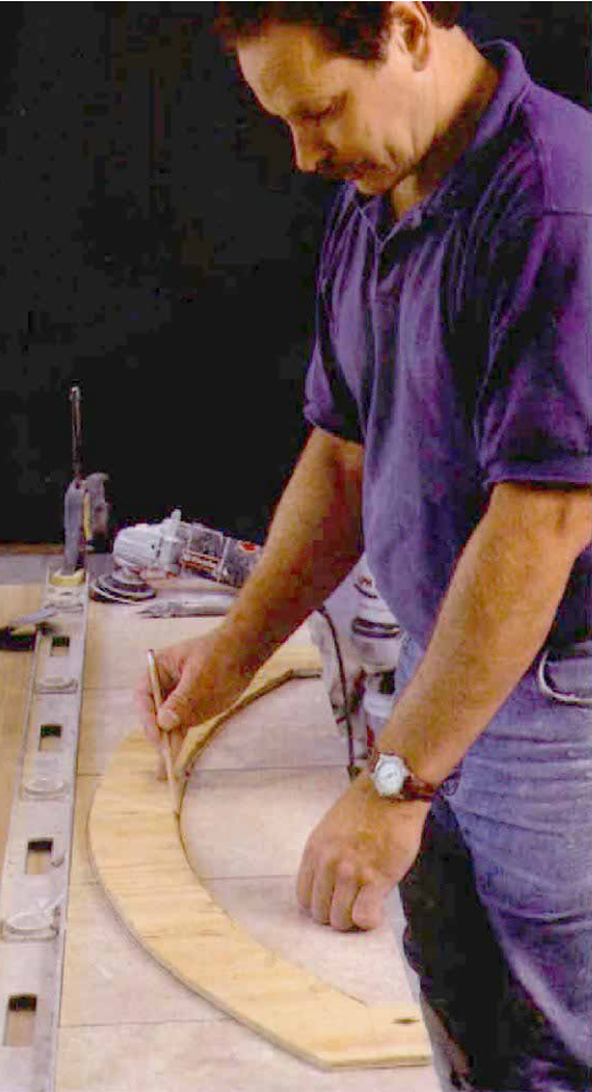
Arched door trim starts with a plywood template. After scribing the arch of the shower entry onto a piece of plywood and adding the top edge of the tile trim, that shape is transferred to the limestone.
