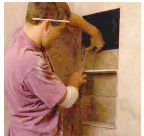
Tiling the niche. After allowing the membrane to cure overnight, the limestone tile is then set into the same latex-modified thinset used in the rest of the room.
